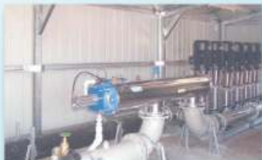
▲ Golf course irrigation, 200µm, Pacific Harbour Golf Course, Bribie Island, Qld, AUSTRALIA
