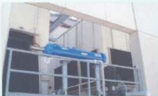
▲ Cooling tower side stream filtration, 100µm, Eastlands Plaza Shopping Centre, Ringwood(Melbourne), AUSTRALIA
