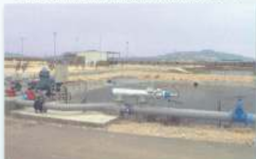
▲ Wastewater reservoir, Pre-filtration to drippers, 400µm, ISRAEL
