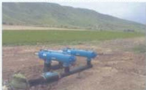
▲ Filtration of well water, Up to 150m³/h, 80µm. Potable water supply system, ISRAEL
